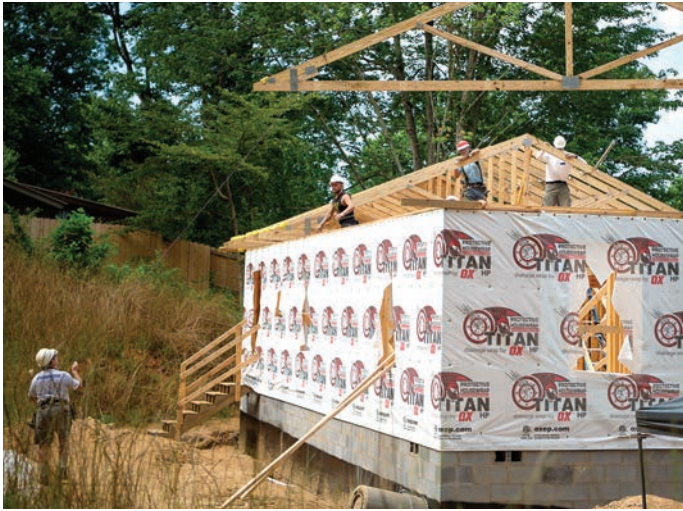
Asheville Habitat staff and volunteers install roof trusses at the jobsite in Mars Hill. The construction of this home was completed in December of last year. ASHEVILLE AREA HABITAT FOR HUMANITY PHOTO
